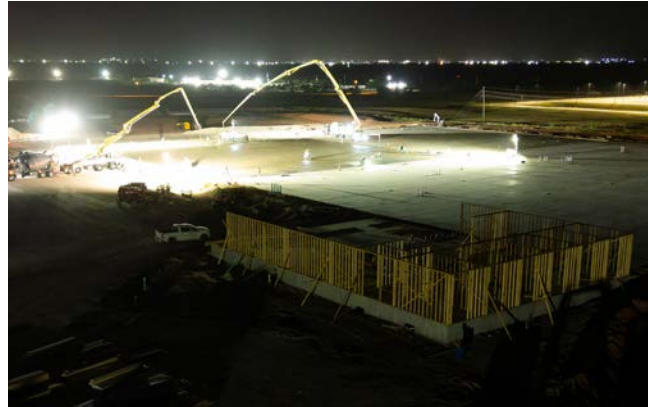
ABI Windows Expansion Project Began pouring concrete for their facility in the DCOA's Five Points Business Park
